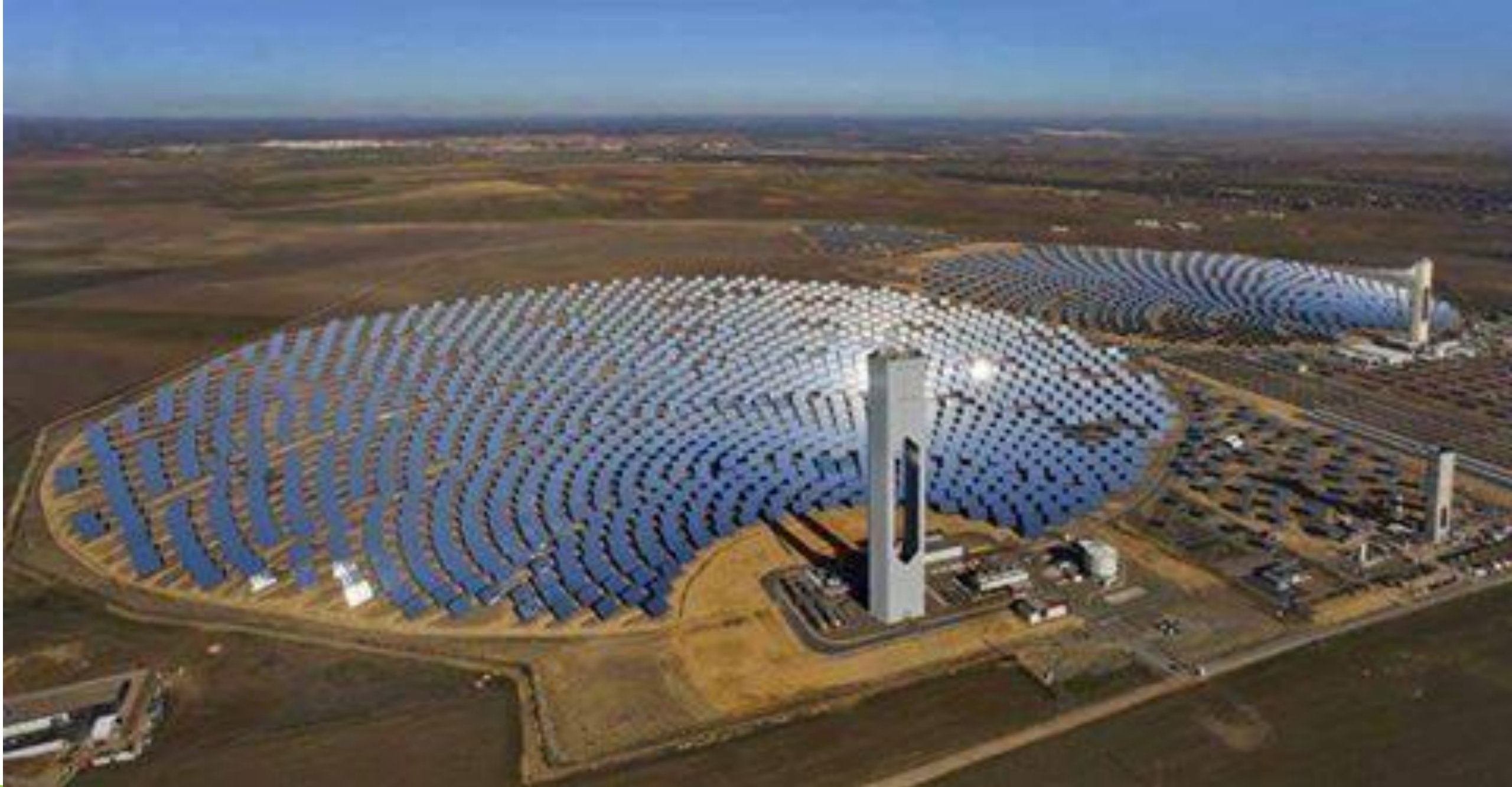
Three hundred megawatt electricity has been added to the national grid after the completion of second phase of the Quaid-i-Azam Solar Park near Bahawalpur
