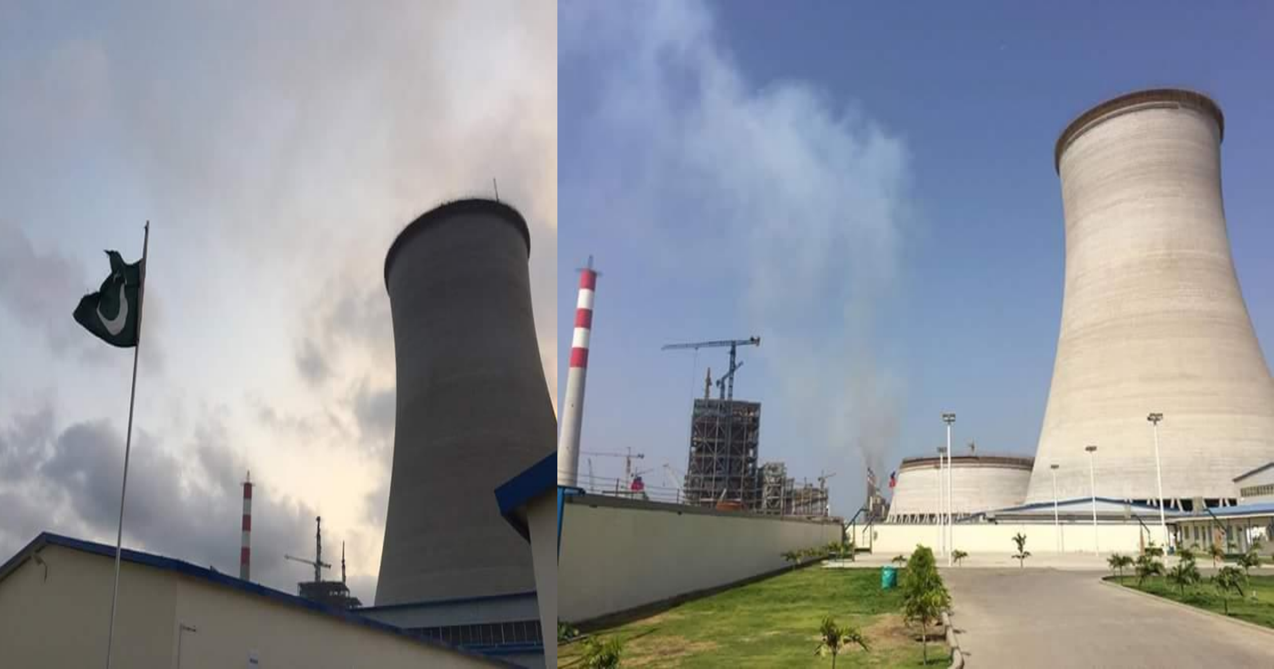
KARACHI: Under-construction 1,320 MW Port Qasim Power Project comprising two 660 MW supercritical coal power plants
